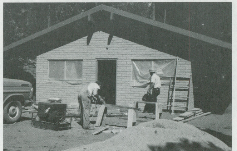
The main washroom at Leoni Meadows will house restrooms, showers, washers and dryers.
