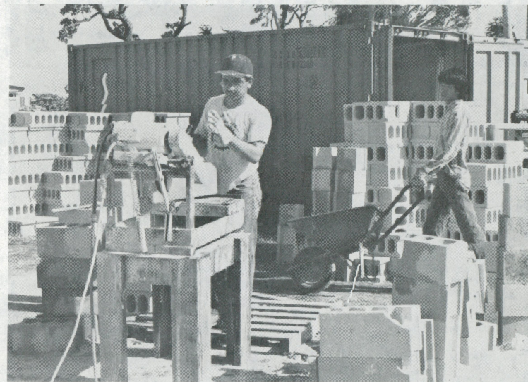
Six shipping containers of building materials preceded San Gabriel students to Majuro—shipped to the specifications of John Clough, retired physical plant supervisor at La Sierra. Now calling Hood River, Oregon, home, Mr. Clough designed the building and supervised construction. The Cloughs have lived on Majuro the past two years. Carlos Garbutt wore out three sawblades during his faithful and meticulous cutting.
