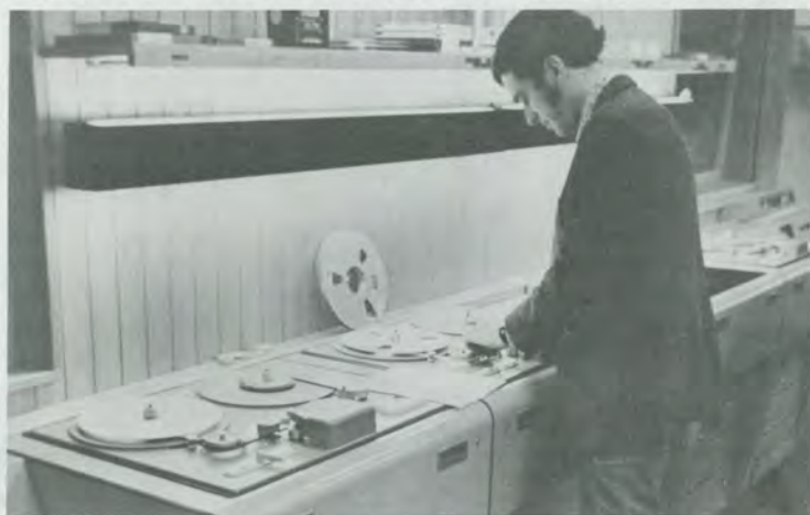
AWR Program Manager Allen Steele in the Sesimbra, Portugal, studio, where the latest equipment guarantees the best possible shortwave signal.
