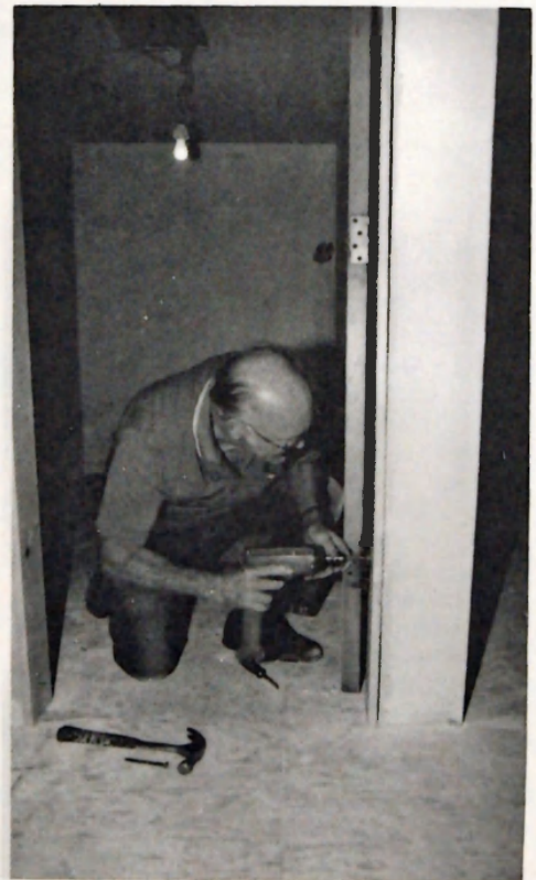
Delbert Bollinger continues the building of the new Teaching Learning Center above the Student Center. Expected date of completion is around the middle of next week. (Sept. 16-22) Photo by Erik Stenbakken
