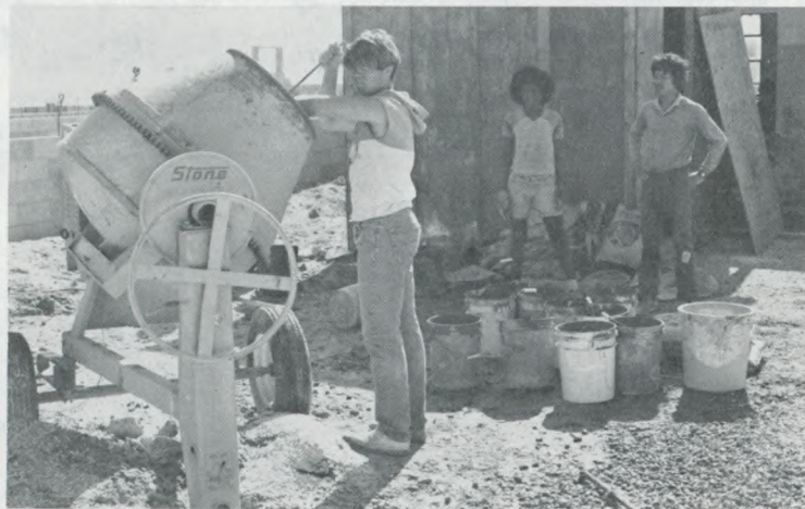
For two weeks Brent Robinson, who took a semester's leave from his studies at East Los Angeles College to join his former schoolmates from San Gabriel Academy, mixed mortar. In fact, he went a week ahead of the group and remains in Majuro today to help finish the building.
