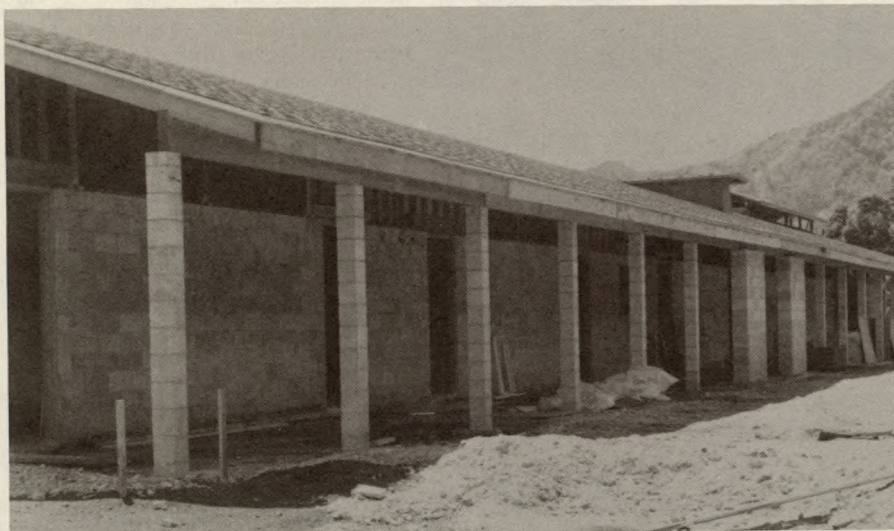
Progress is continuing on the construction of new classrooms at the Kahili Mountain School on Kauai. The buildings must be securely anchored to withstand potential hurricane winds.
