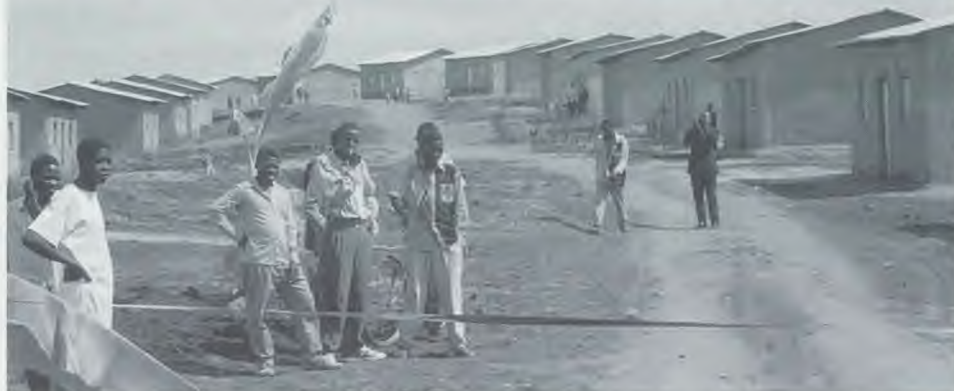
At the Murambi project in Rwanda, ADRA is coordinating the construction of starter houses for families who have been living under plastic sheeting
