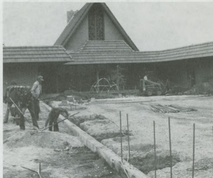
Members of the Campbell Church donate their labor toward making their new sanctuary a reality.
