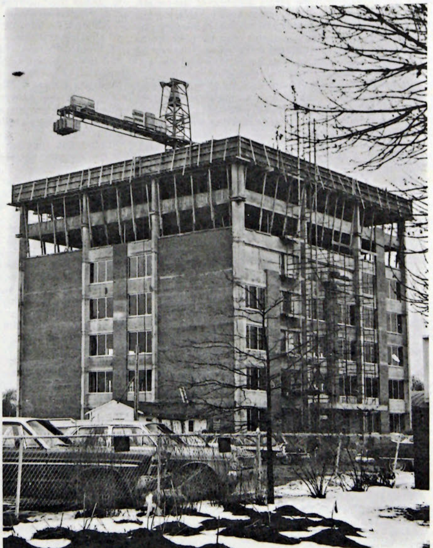
In the winter of 1966, the top two floors of Prescott Hall were exceptionally drafty.
