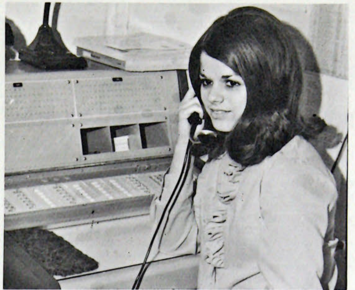
Photo by Gary Bollinger The new pushbutton switchboard, which has recently been installed, makes answering calls easier and more enjoyable for Donna Stone, one of the operators.
