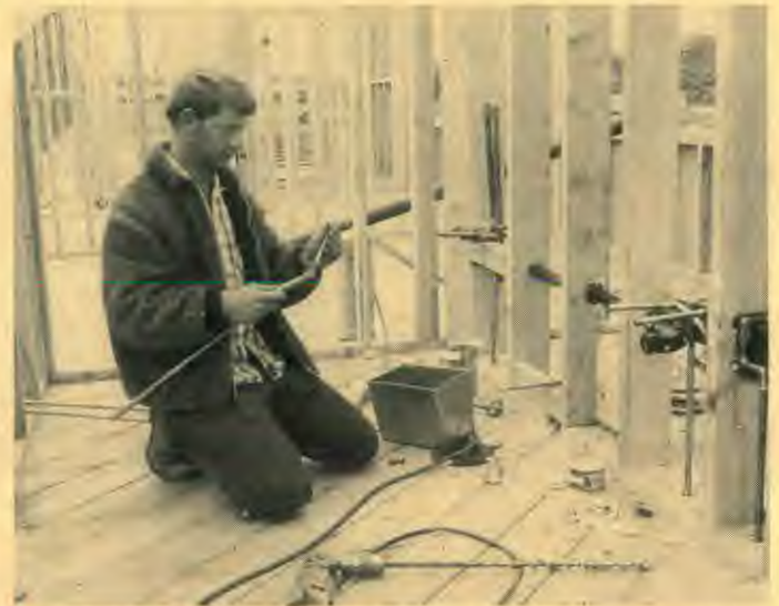
The wiring and plumbing of the east and west wings nearing completion.
