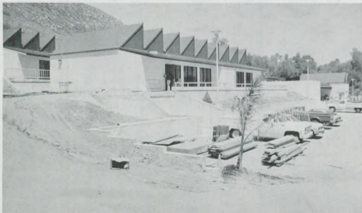
The Visual Art Center on the La Sierra Campus of Loma Linda University is nearing completion, with the grand opening set for October 4.
