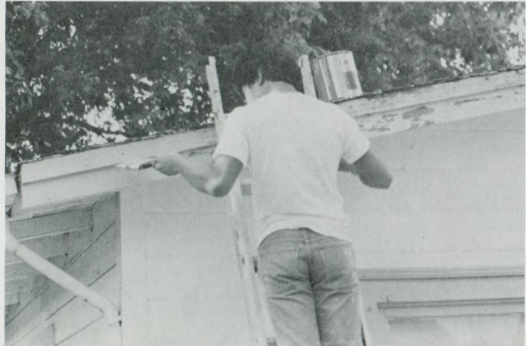
Hayward youth spent several afternoons a week restoring the home of a 78-year-old church member while she was away for two months. Along with painting the exterior, the youth also rebuilt the home's porch.
