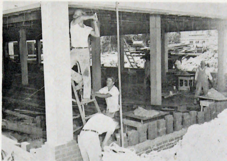
Students help lay brick and construct concrete supports on the new South Hall wing. Plans are progressing toward its completion in September, 1960.
